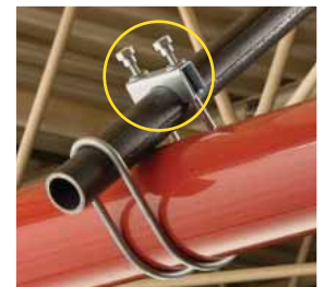
Step 3: Finger tighten the bolts until brace pipe is firmly held in place.
